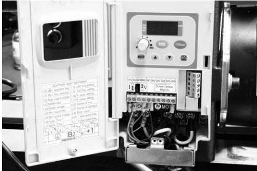
VFD with cover open
