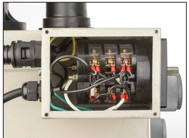
Figure 49. Switch box wiring.
