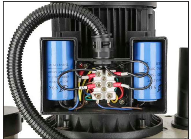
Figure 48. Motor junction box wiring.
