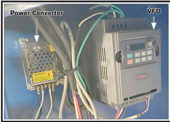
Figure 91. Electrical components inside cabinet.
