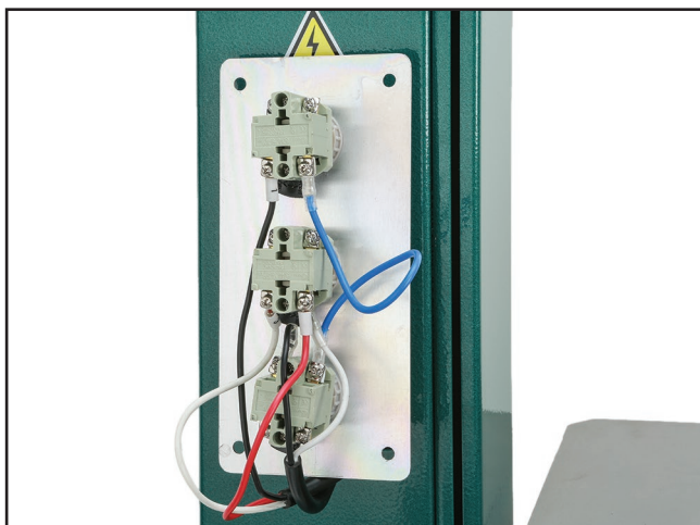
Figure 118. Control panel wiring.
